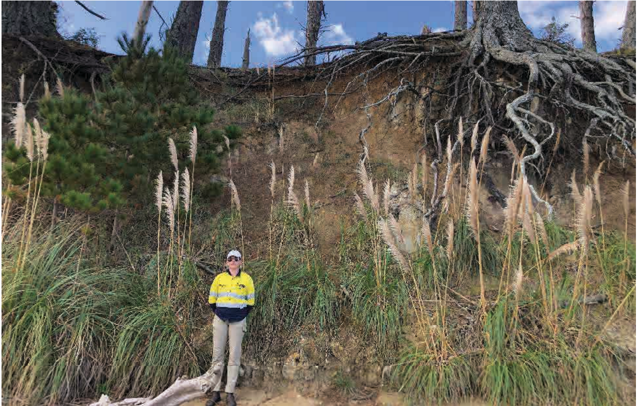
Plate 1. Eroding bluff face adjacent to Grid 1a and 1b, facing north-west. Note shallow layer of midden material is eroding from the uppermost deposits within the root system of the pine trees.
